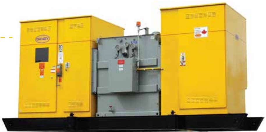
Model #S-PHV-US-34kV-2MVA complete with primary disconnect, 34,500V transformer and 4160V secondary sub distribution
